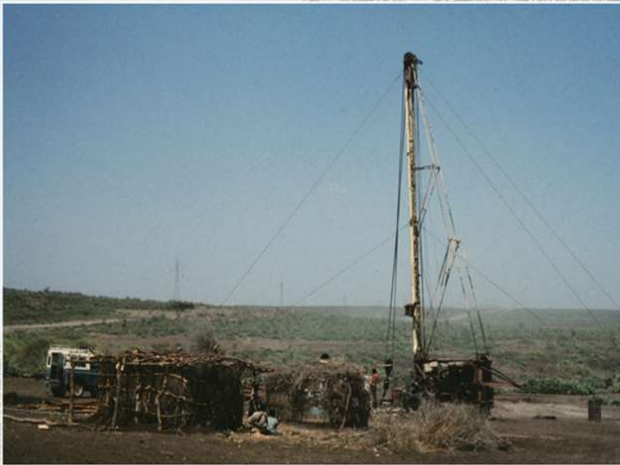
Cable tool-drilling rig near Beseka Lake. Percussion drilling of 100 meters deep hydrogeological borehole in hard basalts of Afar Depression. It took several months to undertake this activity.
